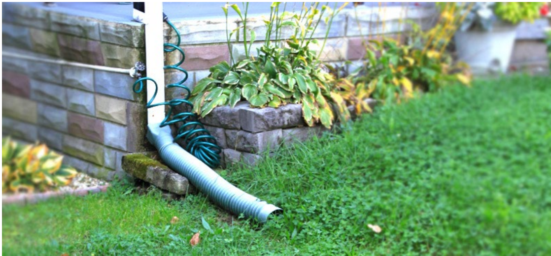
Figure 35 Disconnected downspout in a yard
