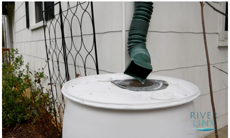
Figure 25 Downspout directed into rain barrel
