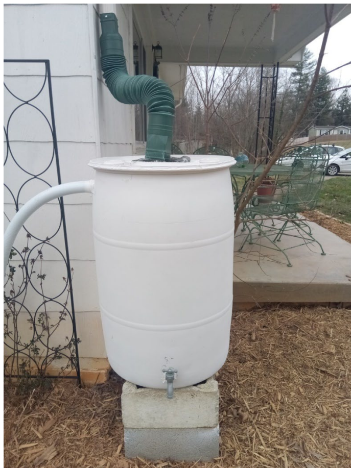
Figure 17 Installed rain barrel
